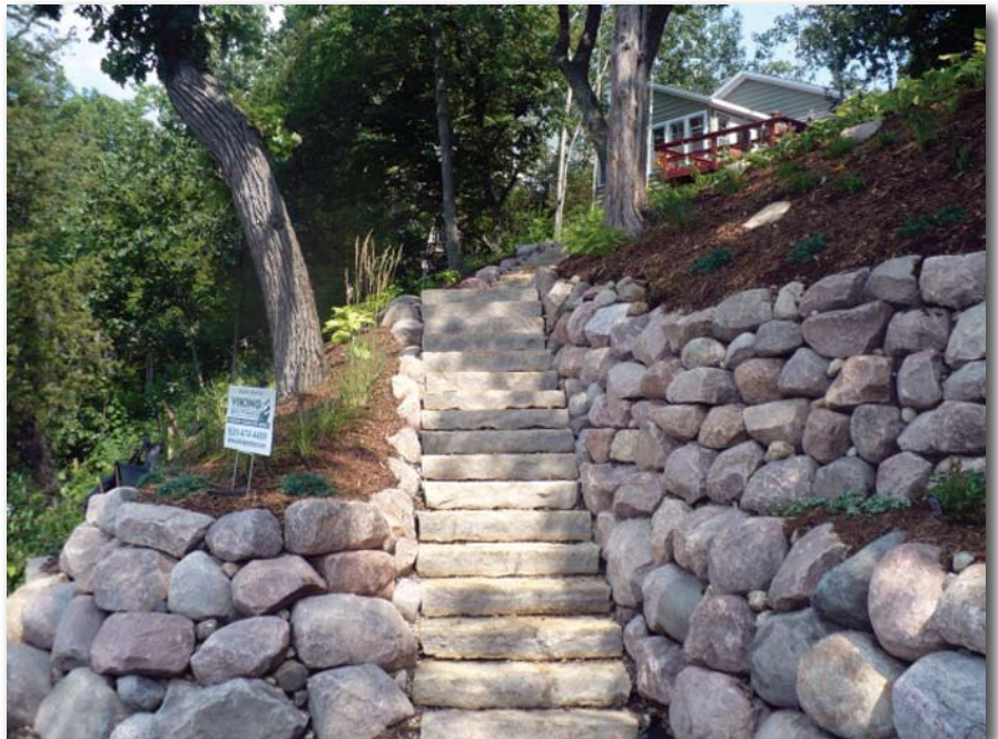
A clear view of the completed retaining wall and Lemke stone steps.
